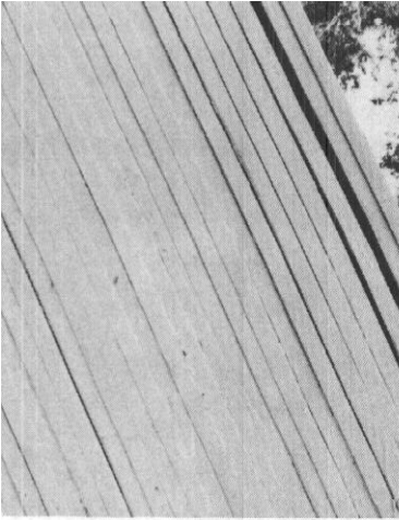
Figure 4-5. Glulam arches with rating 40. (A) Severe delamination in a localized area in the outer laminations.
