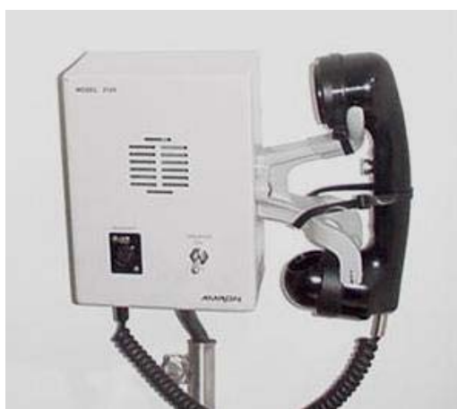
Figure 2-10. Interior Communications Panel
