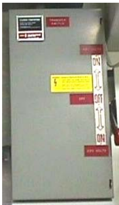
Figure 3-2. Manual Bus Transfer (MBT) Switch
