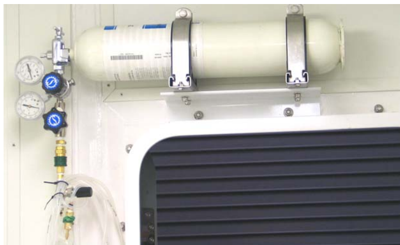
Figure 2-13. Calibration Sample Gas Cylinder
