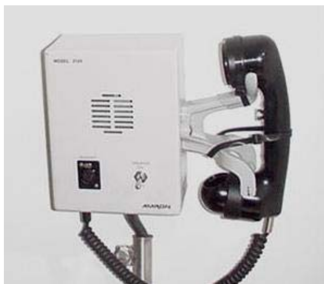
Figure 3-17. Interior Communications Panel
