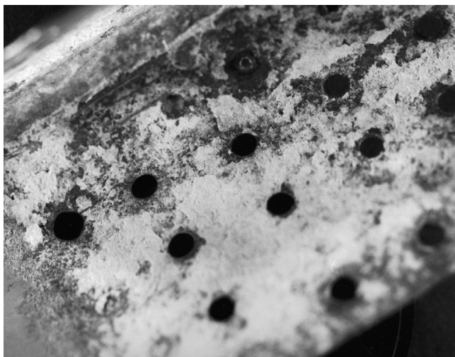
Figure 3-23. Aluminum Surface Corrosion Products
