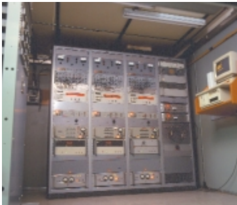
Figure 3.6. WWV Control Room
