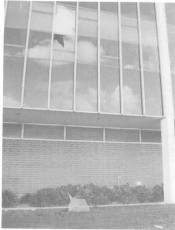
Earthquake Damage: 1994, Northridge, California Photo Credit: Wiss, Janney, Elstner Associates, Inc.
