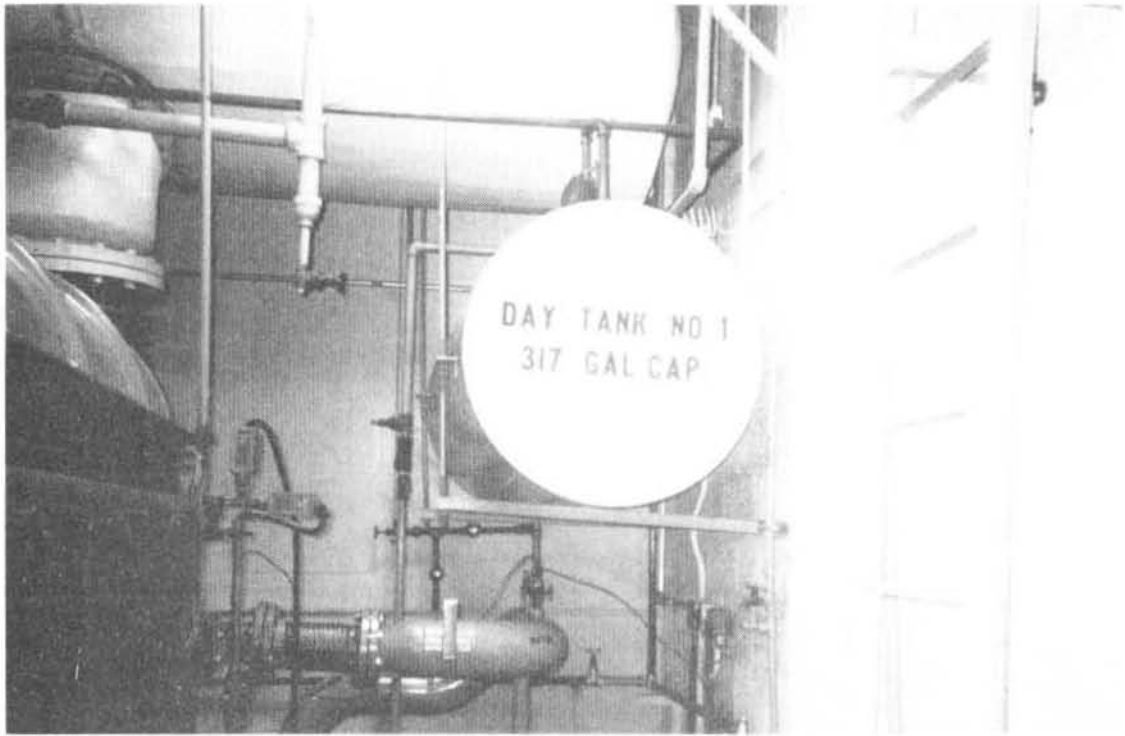
Unbraced Day Tank, Hospital, Puerto Rico Photo Credit: Wiss, Janney, Elstner Associates, Inc.
