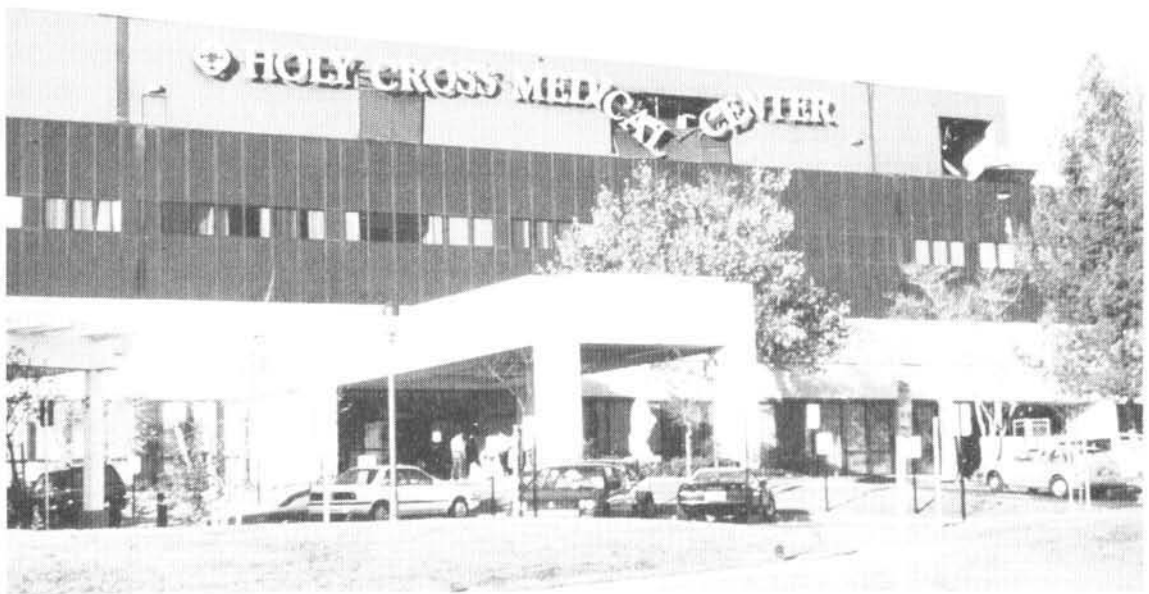
HVAC damage at Holy Cross Medical Center in Sylmar—damage to signage and louvers caused when suspended fans in the mechanical penthouse swung and impacted the louver panels. HVAC service outage caused the temporary evacuation of all patients. Earthquake Damage: 1994, Northridge, California Photo Credit: Robert Reitherman
