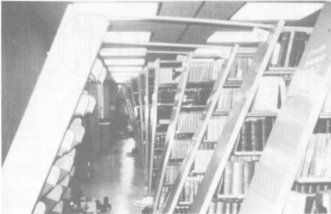
Failure of inadequately upgraded library shelving Earthquake Damage: 1987, Whittier Narrows, California Photo Credit: Earthquake Engineering Research Institute, Marshall Lew & Greg Brandow C12b
