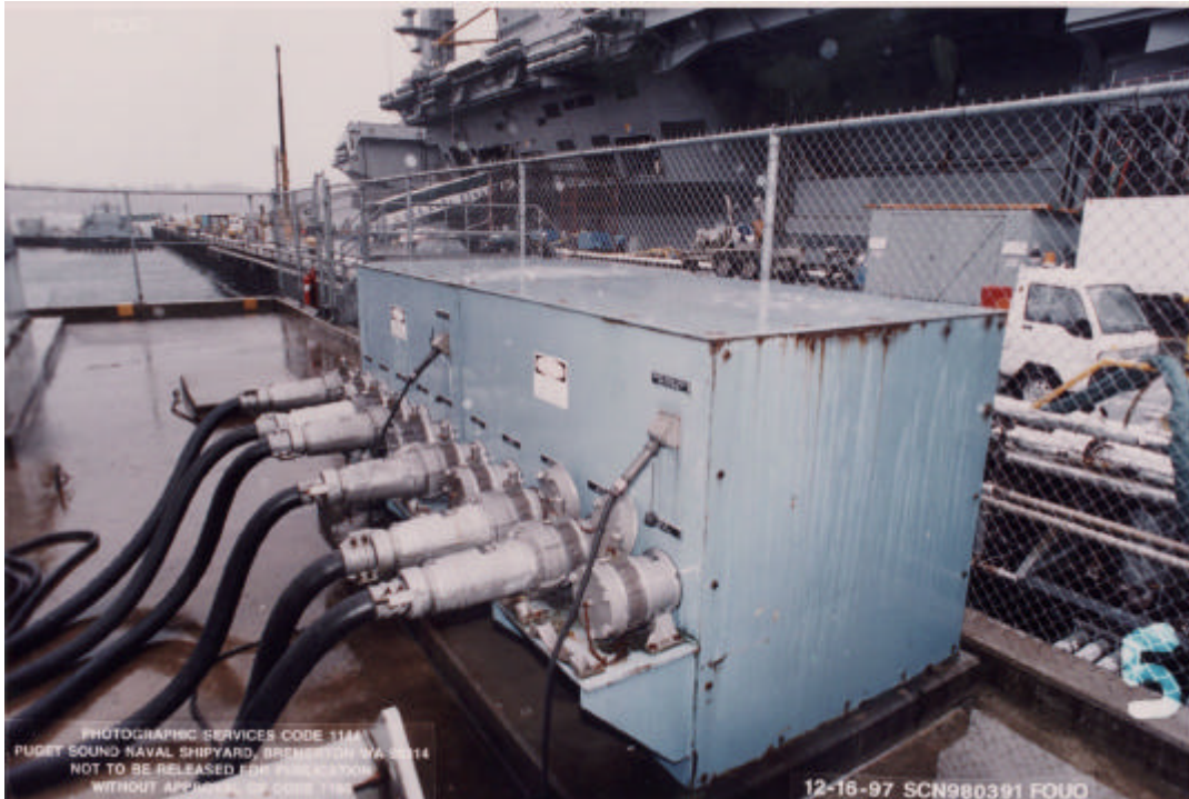
Picture F. A 4.16-kV pier electrical outlet assembly and outlets.
