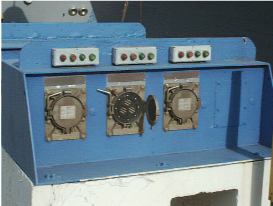
Picture E. A 480-volt pier electrical outlet assembly without cable connections.
