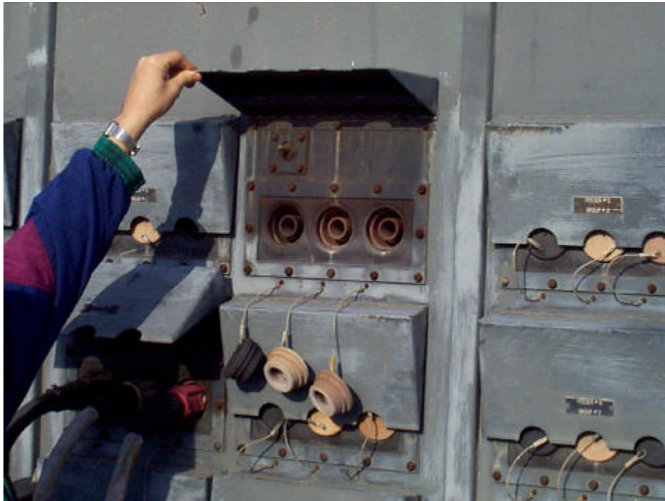
Picture D. A skid-mounted substation with camlock connections.
