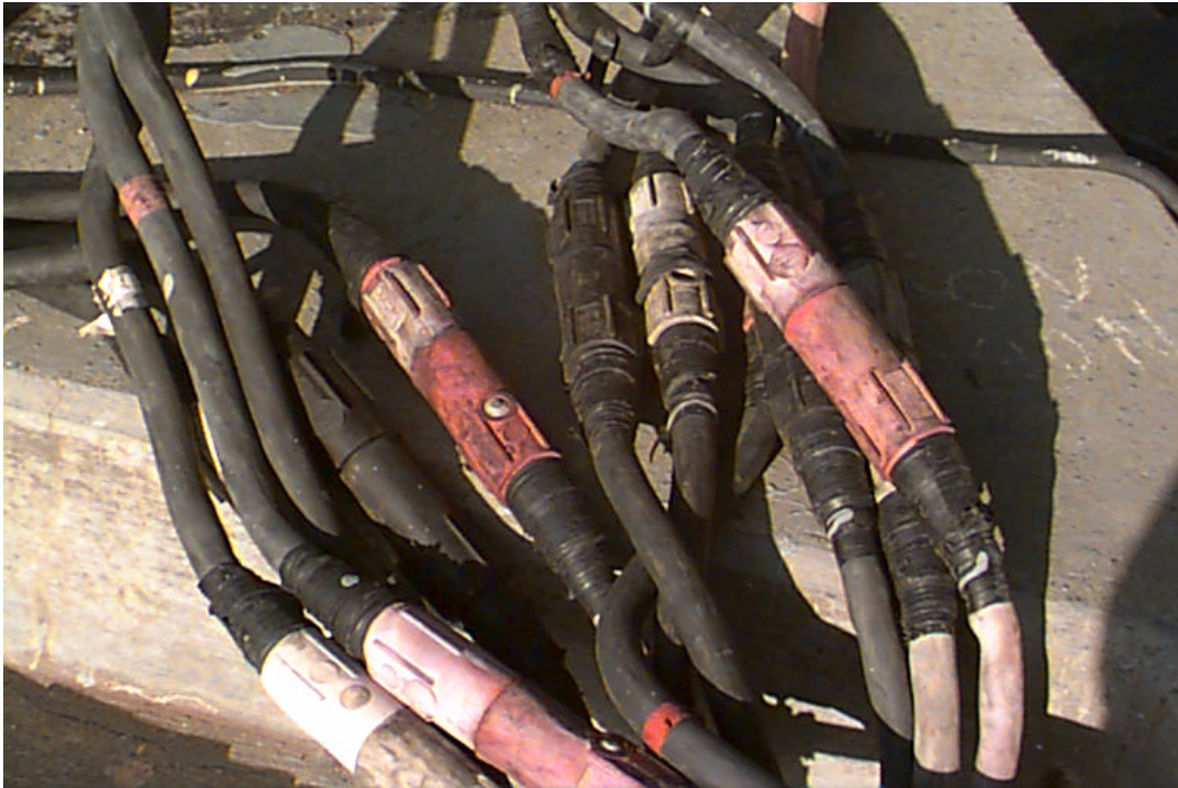
Picture I. A 480-volt shore-cable to ship-cable with camlock connection.
