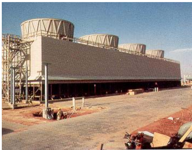
Figure 4-9. Counter-Flow Cooling Tower
